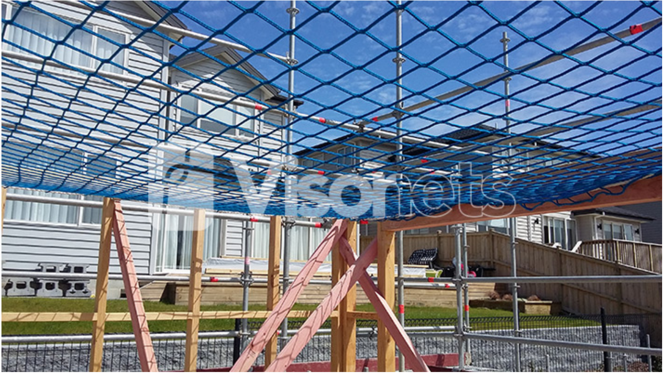
Example of safety net installed in residential housing in NZ.
